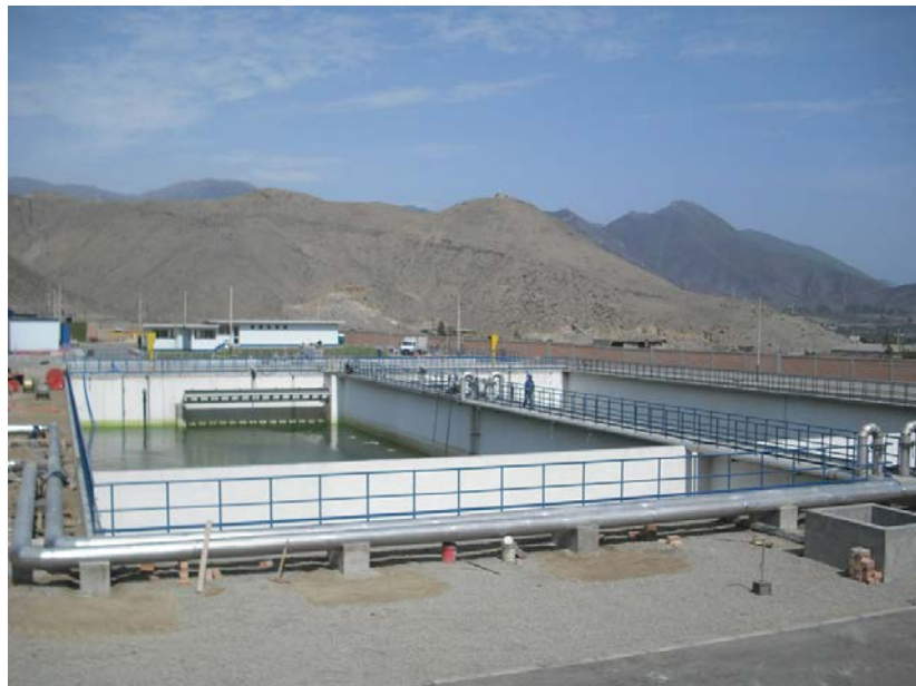
As soon as the regional water balance is modelled, innovative management approaches will be prepared, which should contribute to sustainable water supply and wastewater disposal in Lima even after the project has ended. Photo: Christian León
